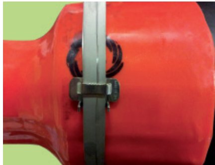
2. Fix included steel straps on the front end of the seal on the casing pipe side.
