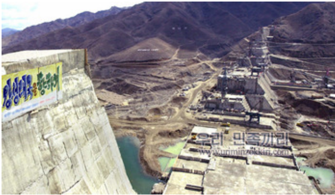
Construction site of a dam in Jagang Province. The slogan on the left reads “Towards a Powerful Country.” [Picture: Uriminjokkiri]
